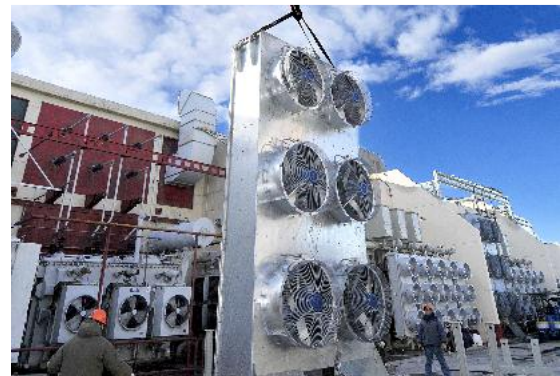
Cooling upgrade designed and implemented to match new operation conditions
