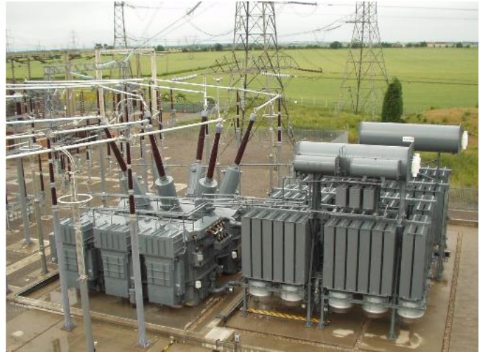
Quadrature Booster 2750 MVA 400/80 kV for National Grid Co. plc. High Marnham (UK)
