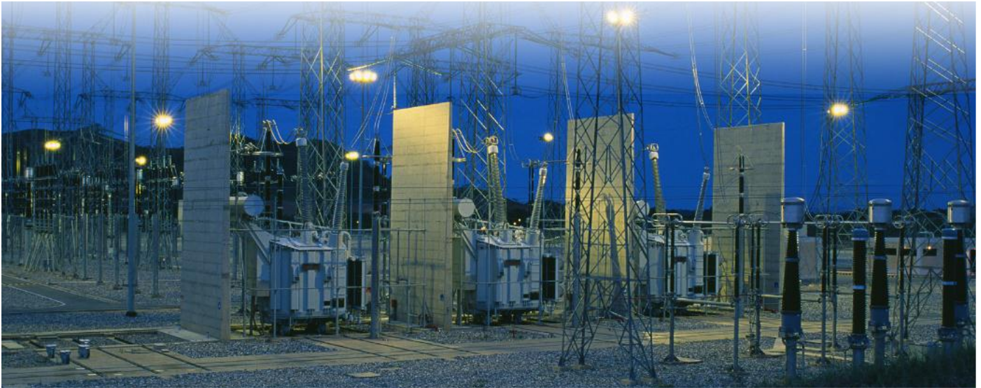
Single-phase autotransformers 500 MVA 765/400/20 kV in operation since the early 80's for EDELCA (Venezuela)
