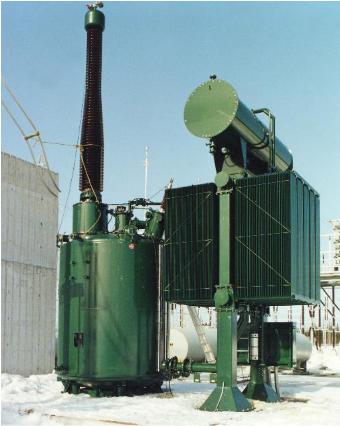
110 Mvar, 765 kV single-phase shunt reactor for Hydro Quebec. Chamouchouane s/s (Canada)
