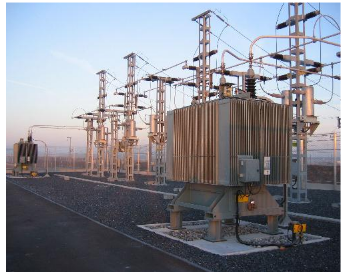
Autotransformers in SNCF railways (France)
