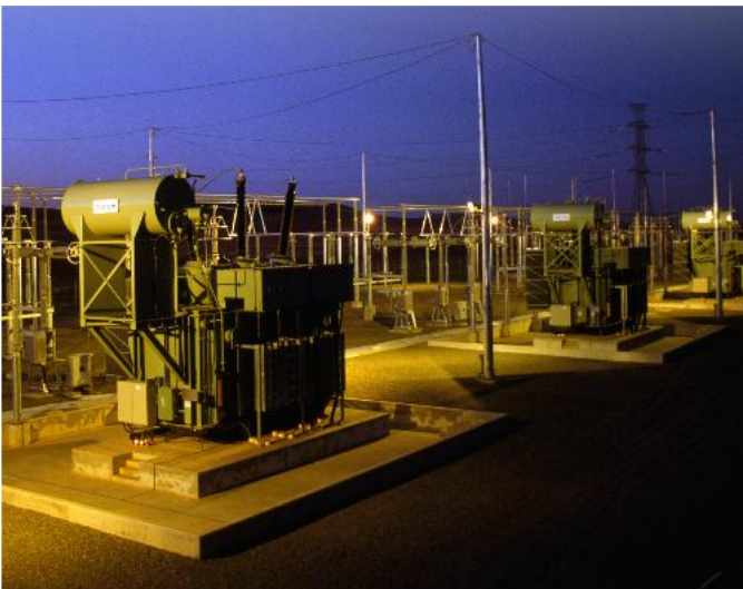
Generator transformers 100 MVA 275/13,2/13,2 kV for AGL, Hallet power plant (Australia)
