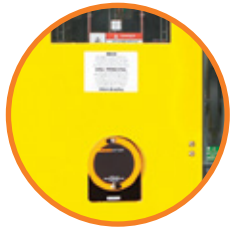
1 Yellow door – helps identify main disconnect for MCC lineup
